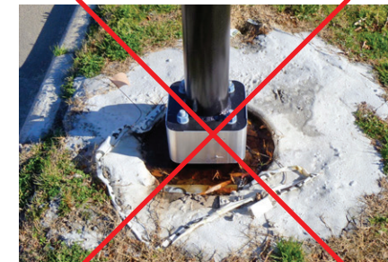
Unacceptable Footer Detail
