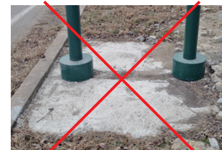
Unacceptable Footer Detail
