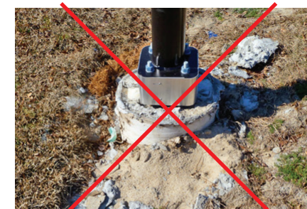
Unacceptable Footer Detail
