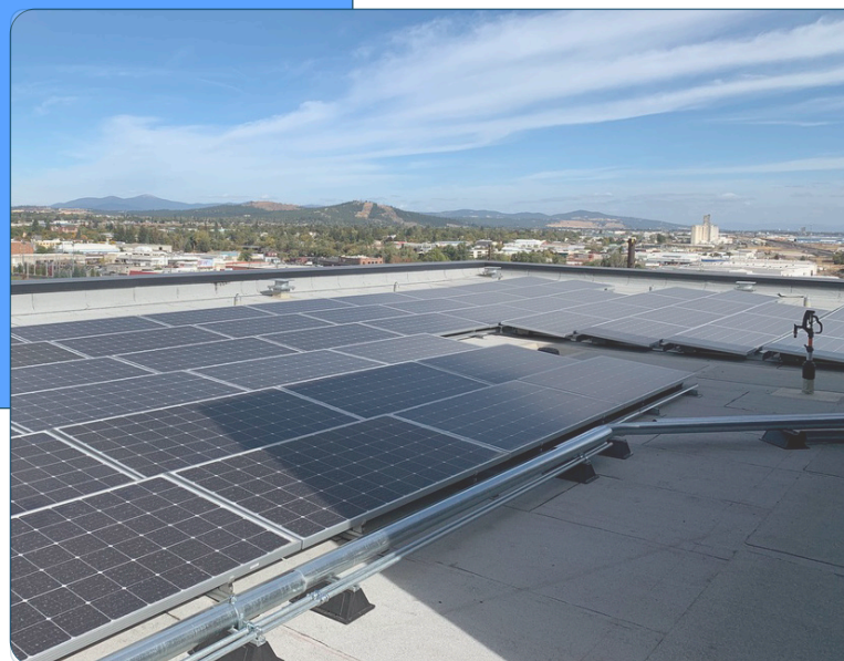
Rooftop solar array in UD
